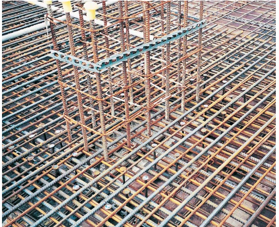
Figure 1: Loose bars laid around starter bars for column, where shear heads are in position.
